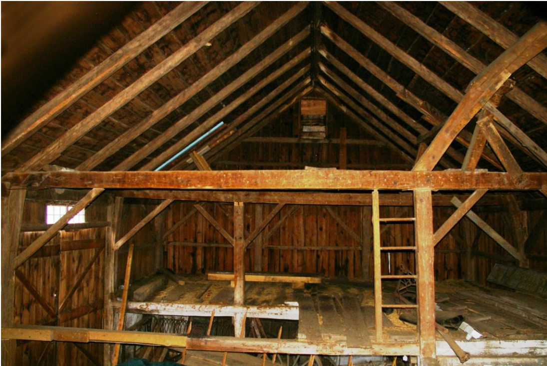
TIMBER FRAMING FAILURE: The post and two braces at the hayloft, beyond the threshing floor, have dropped and their connection to the girt above has completely failed, due to a post removed from the girt below, resulting in substantial sag over a long span.
