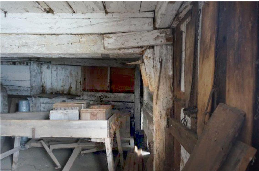
POST TO GIRT CONNECTION FAILURE: The post to girt connection has failed, with a second timber added below the original girt, a blocking added where the timber meets the post, and a spline
